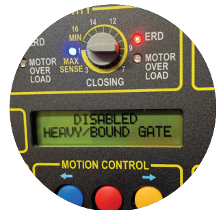
Heavy gate or binding gate detected
